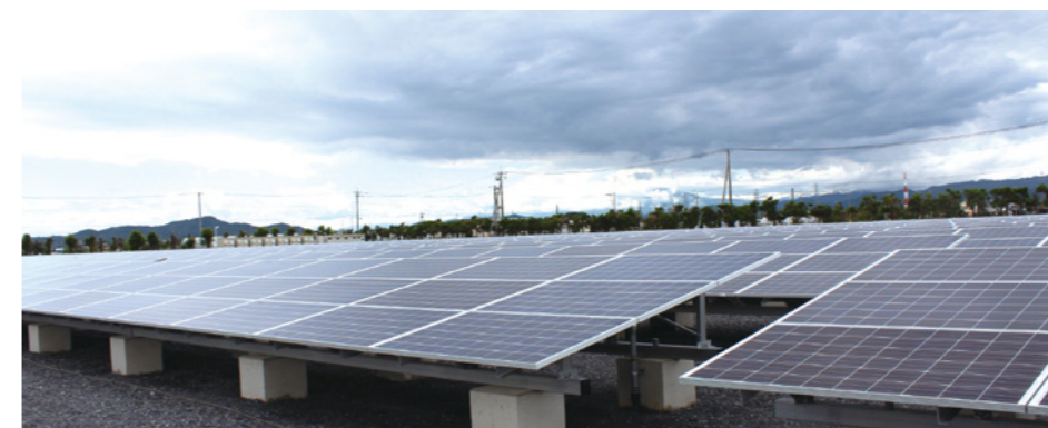
Solar panels at the BANDO eco moving solar power facility
