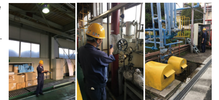
Inside Nankai Plant (Measurement of illuminance/temperature/power)
